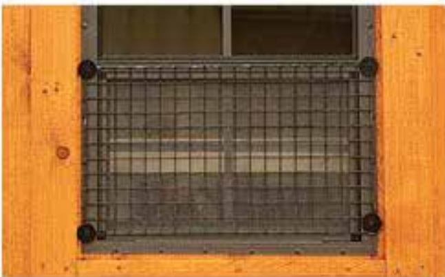
Wire over window
